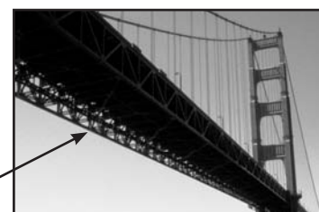
Fig. 49 - The use of trusses on the road decking of a suspension bridge.
